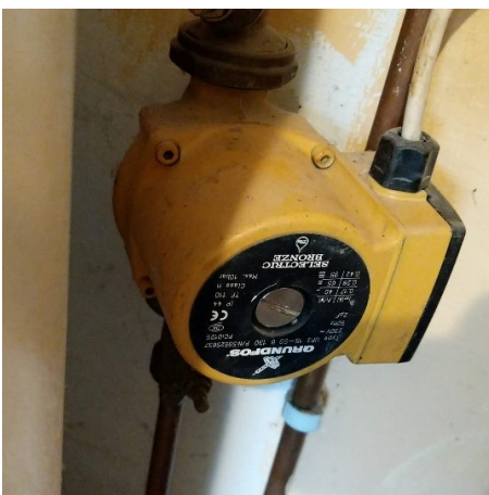
Secondary circulation system pump
